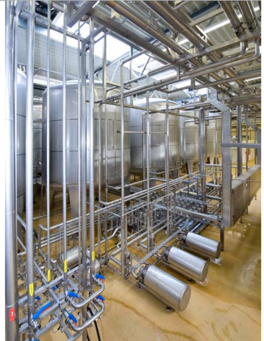
Concentrate pumps and containers
